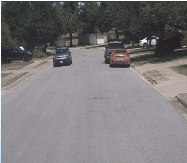
GREENING WAY (PCI=96.9, Good Condition)
