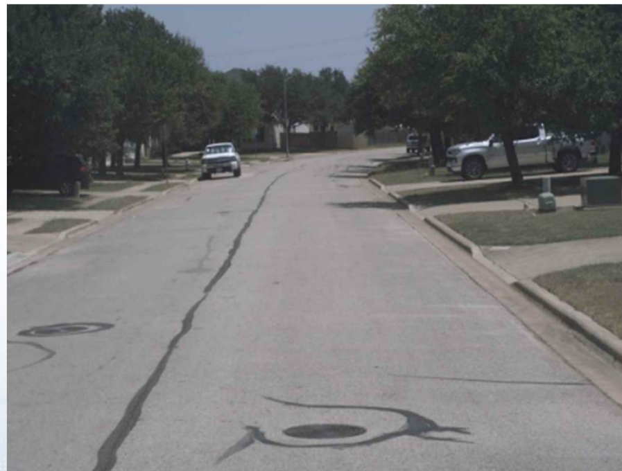
MCCARTHUR DR (PCI=76.9, Satisfactory Condition)
