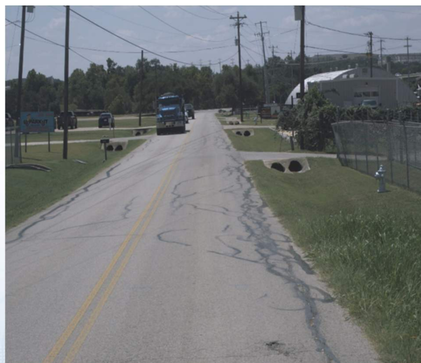
CR 269 (PCI= 41.2, Poor Condition)
