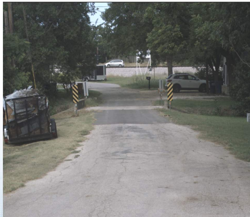
E EVANS ST (PCI=21.3, Serious Condition)
